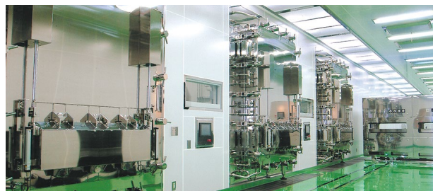
Freeze dryers and automatic guided vehicles (AGV)
