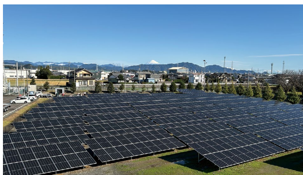
Solar Power Generation (Fujieda Site)
