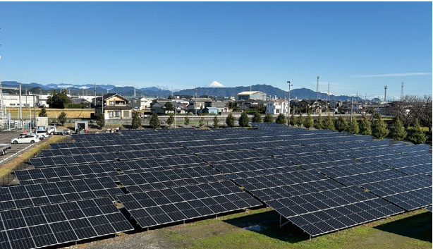
Solar Power Generation (Fujieda Site)
