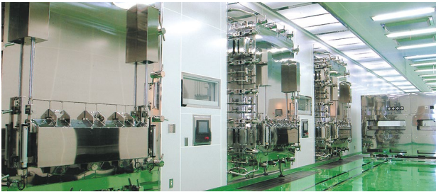
Freeze dryers and automatic guided vehicles (AGV)
